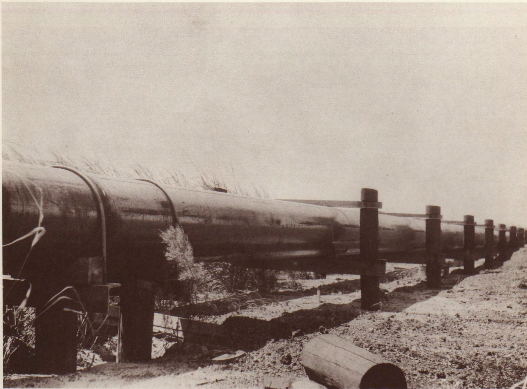
DUAL PIPE CIRCULATION LINE, OKLAHOMA GAS & ELECTRIC COMPANY Harrah, Oklahoma
