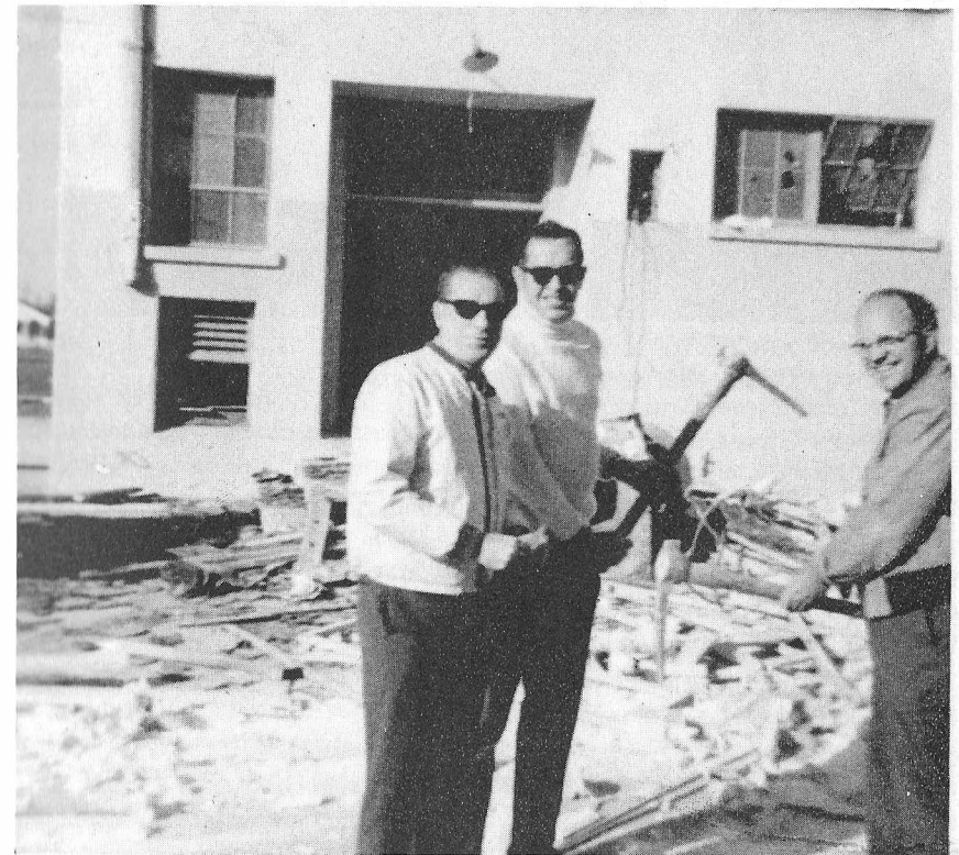
THE OLD GIRLS' GYM, having been declared a hazard in the event of an earthquake, did not give up easily as the heavy equipment tackled the demolition. Watching the action are Harry Strubbe, vice-principal (now director of Adult Education), Dr. Alex Rudoff, principal, and Kenneth Smith, local director of Regional Occupations Program.
