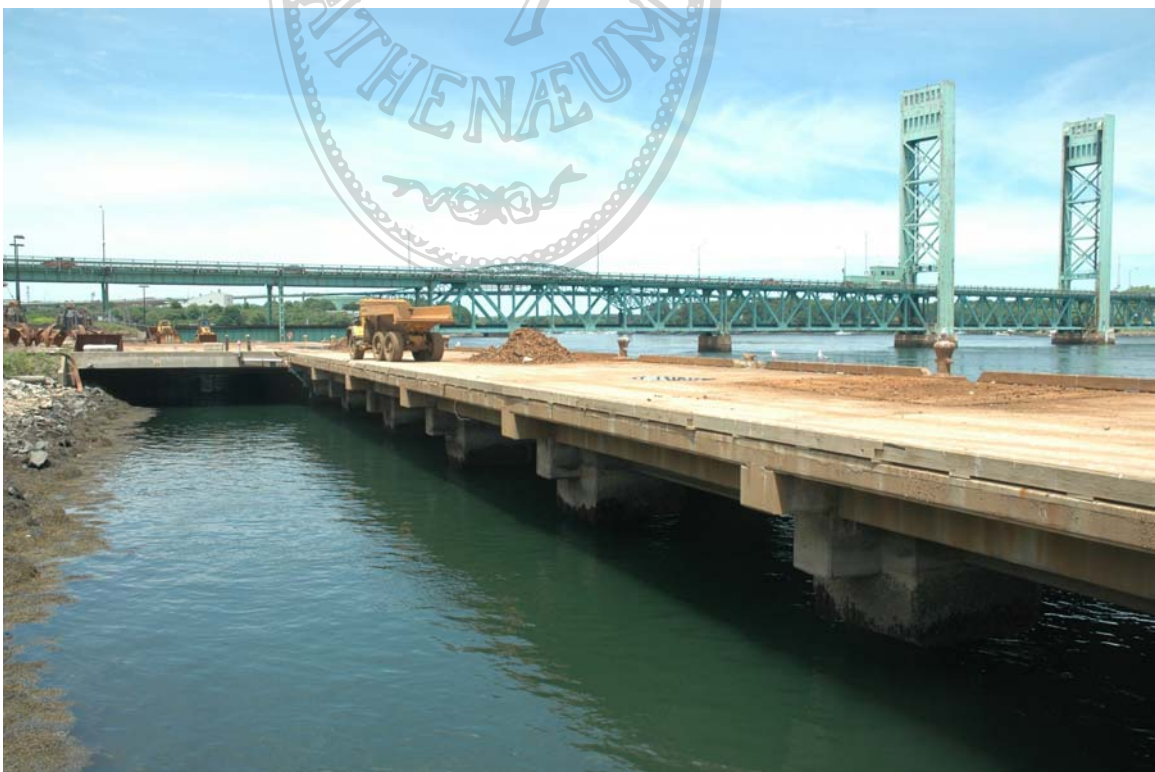
Photo 31) Concrete wharf on northeast side of island along Piscataqua River Direction: NW Digital File: ME-NH_0031
