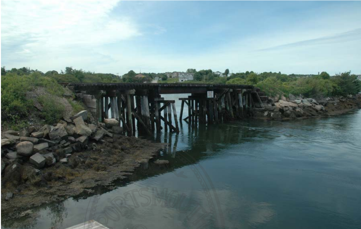
Photo 23) Railroad trestle and berm, northwest of Sarah Mildred Long Bridge, from Nobles Island to Freeman's Point Direction: W Digital File: ME-NH_0023
