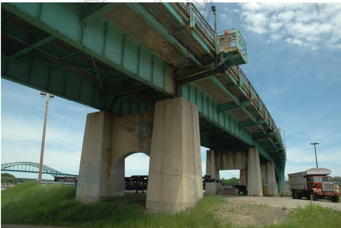
Photo 35) Route 1 Bypass/Sarah Mildred Long Bridge approach on island Direction: N Digital File: ME-NH_0035
