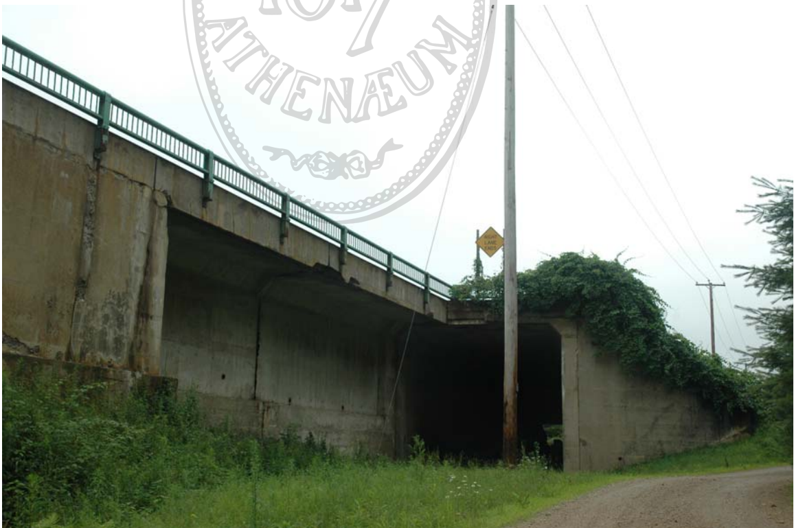
Photo 79) Railroad tunnel and right of way, westerly side of US Route 1 Bypass Direction: S Digital File: ME-NH_0079
