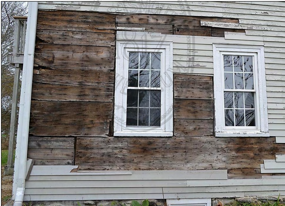
Dennett House, southwestern corner, camera facing north. The exposed sheathing bears a combination of forged and cut nails, with the latter predominating. Cuts in the sheathing above the windows indicate that the windows were lowered or reduced in size at some time.
